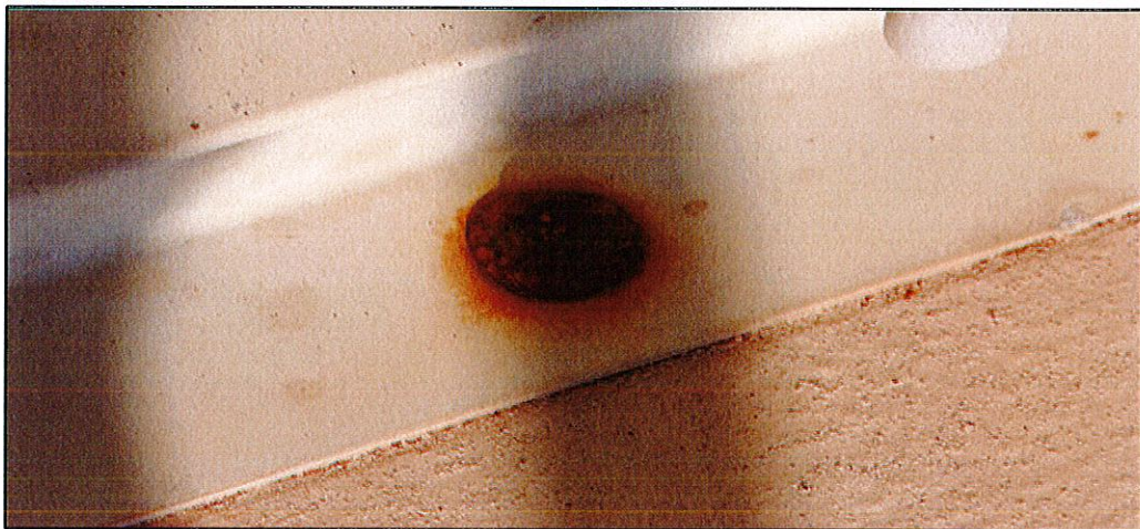
Photo #14. Close up view of deteriorated metal anchors for the hurricane shutters. (Unit 503 shown).
