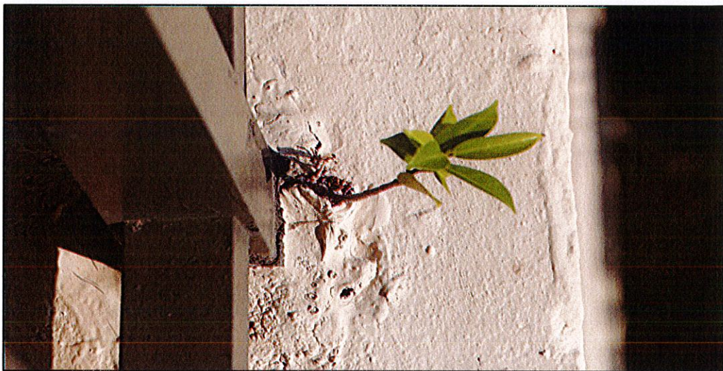
Photo #4. View of post base deteriorated grout and vegetation growth (unit 506 front corridor).
