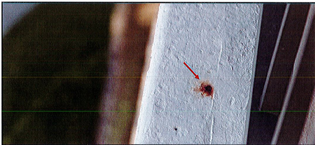
Photo #7. View of exterior stucco finishes with localized bulging and embedded metals with corrosion stains (unit 501 front corridor).
