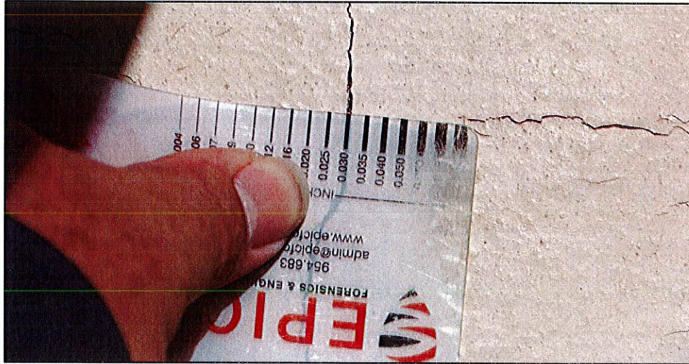
Photo #13. View of medium slab cracks at floor slab (unit 303 front corridor shown).
