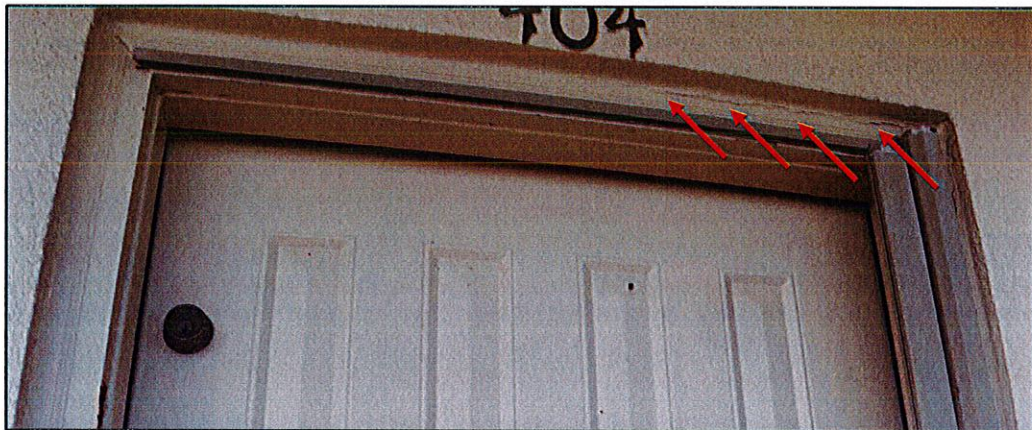
Photo #8. View of deteriorated sealant around the front door of unit 404.
