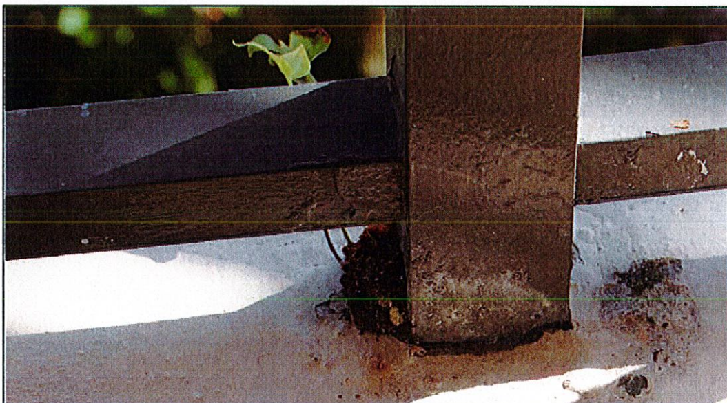
Photo #2. View of post base deteriorated grout and visible vegetation growth (unit 204 front corridor).
