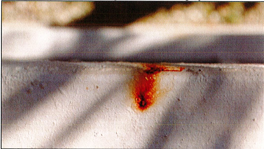
Photo #10. Close up view of embedded metals within concrete slabs with visible corrosion stains (unit 302 front corridor).
