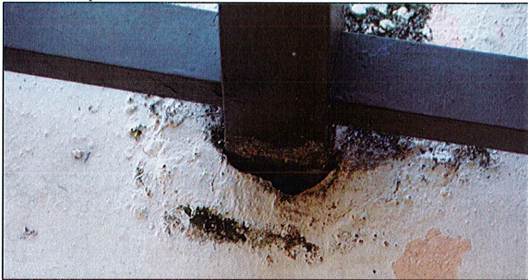
Photo #1. View of post base deteriorated grout with large gaps and metal post with signs of corrosion damage (unit 201 corridor).
