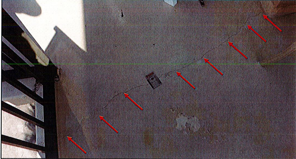
Photo #11. Close up view of embedded metals within concrete slabs with visible corrosion stains (unit 501 balcony shown).
