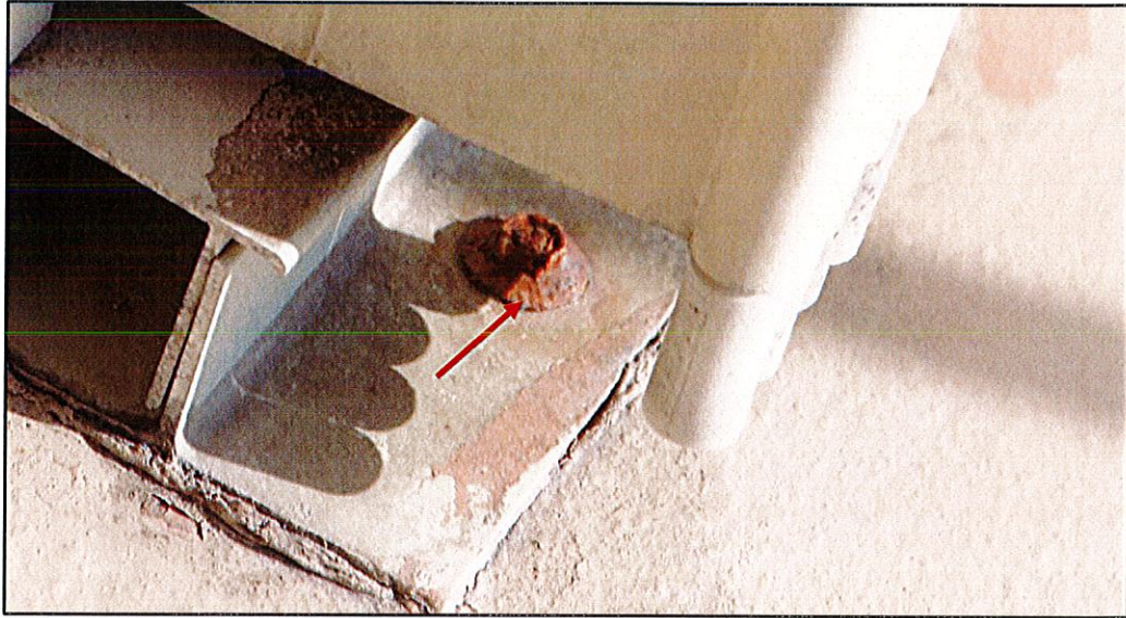
Photo #7. View of deteriorated metal anchors for the hurricane shutters. Observed at several units (unit 405 shown).
