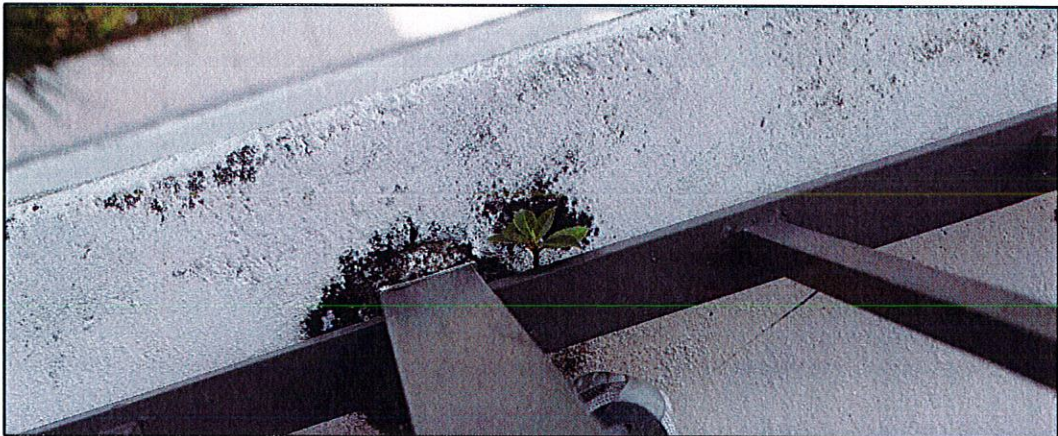
Photo #2. View of post base deteriorated grout and signs of organic growth (unit 506 balcony).
