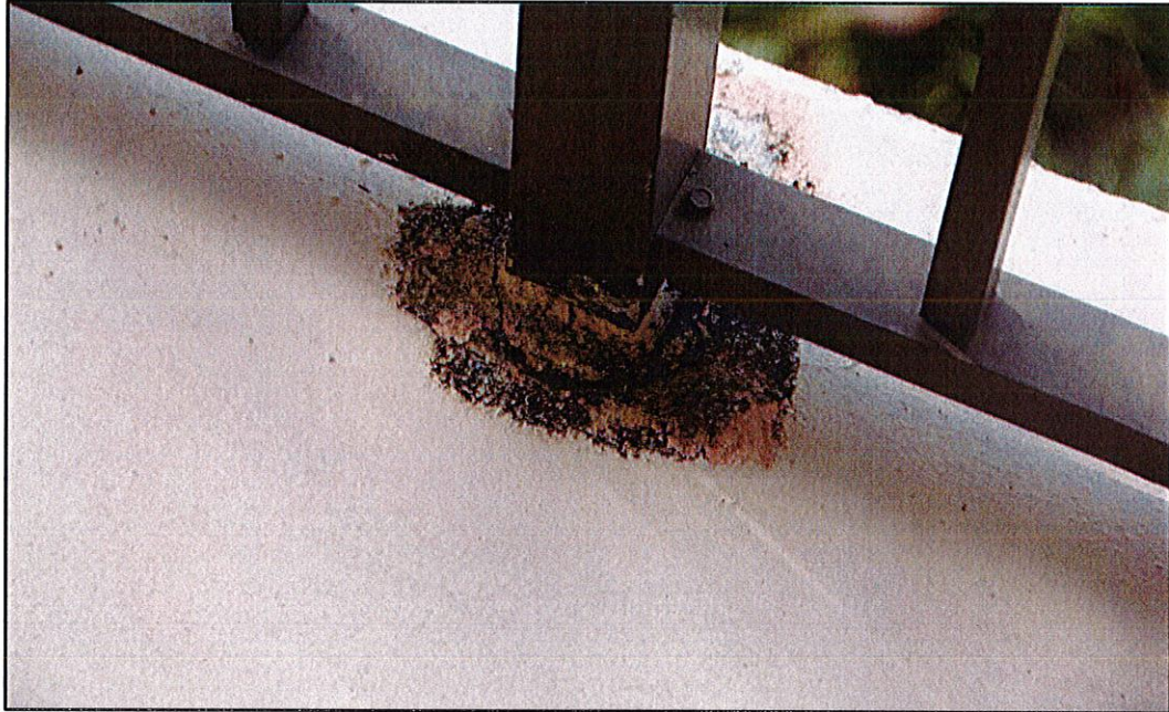
Photo #1. View of post base deteriorated grout and metal post with signs of corrosion damage (unit 402 front corridor).
