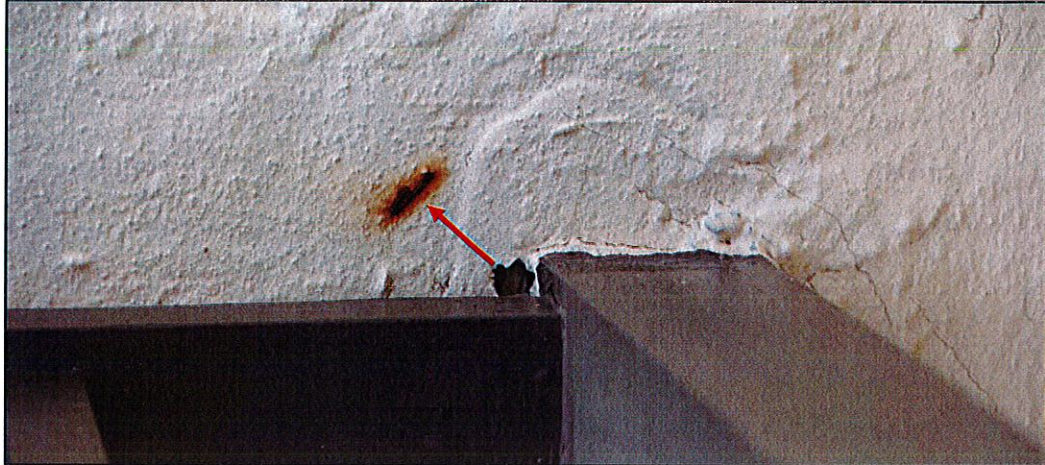
Photo #9. Close up view of embedded metals within concrete slabs. (Unit 501 balcony shown).
