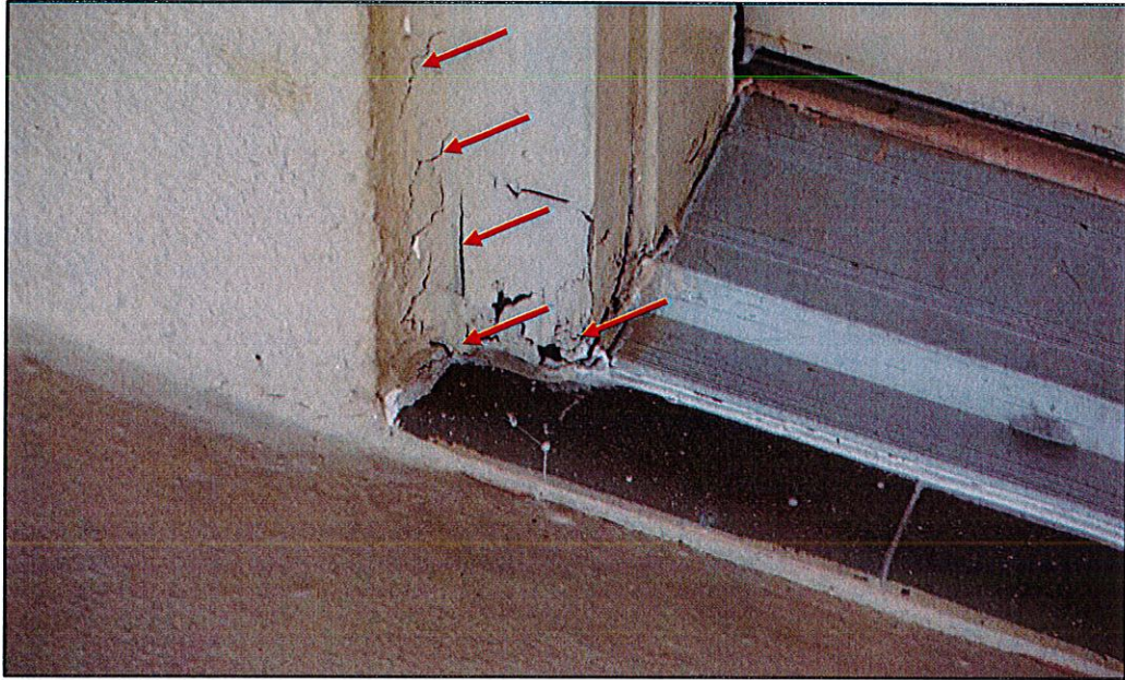
Photo #7. View of deteriorated sealant around the front door of unit 501.
