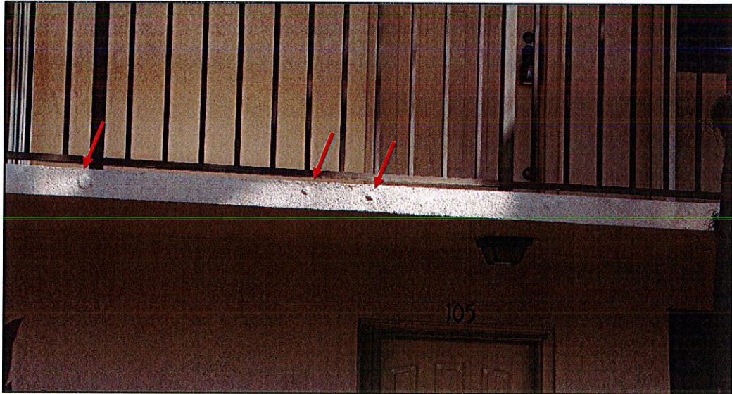
Photo #5. View of exterior stucco finishes with localized bulging (unit 205 front corridor).
