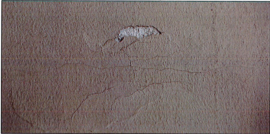
Photo #20. Close up view of slab crack and finished spalling exposing concrete below (Unit 204 front corridor shown).
