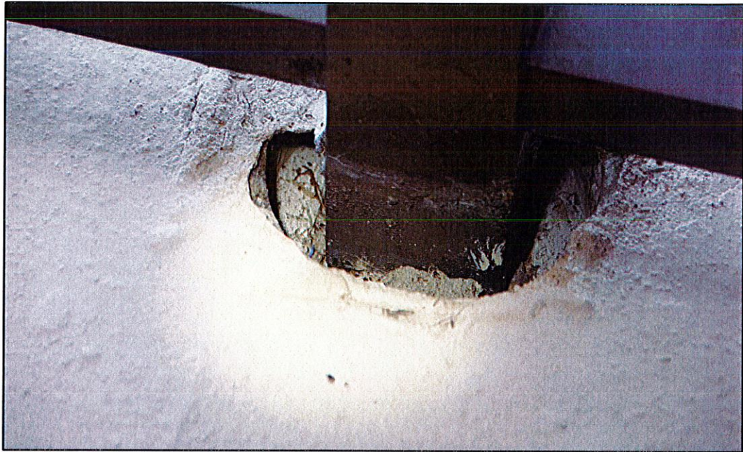
Photo #2. View of post base missing grout (unit 205 front corridor).
