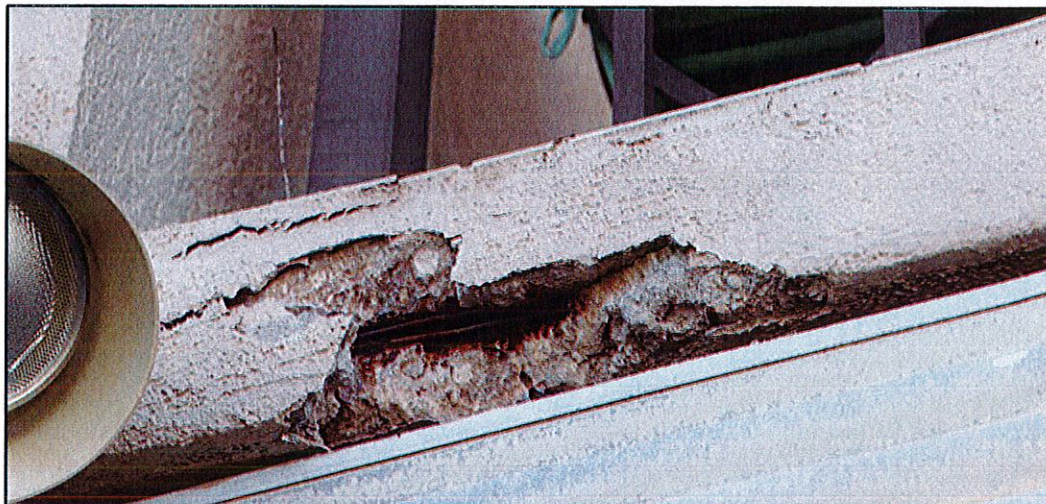
Photo #7. View of imminent spalling of concrete slab edge with corroded reinforcing bars observed at edge of floor (unit 103 balcony shown).
