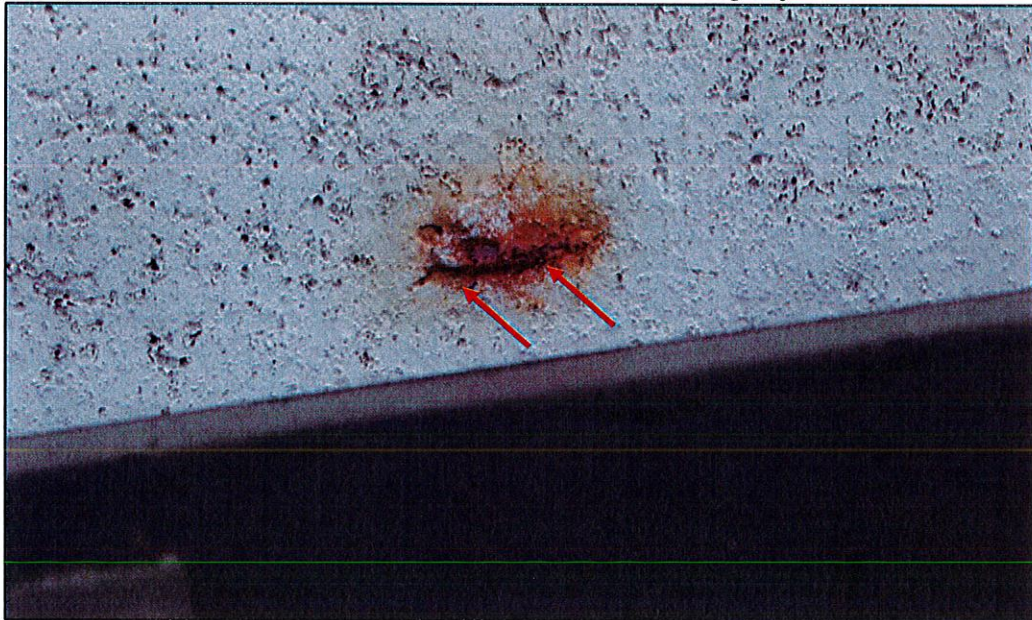
Photo #14. Close up view of embedded metals within concrete slabs. (Unit 506 balcony shown).
