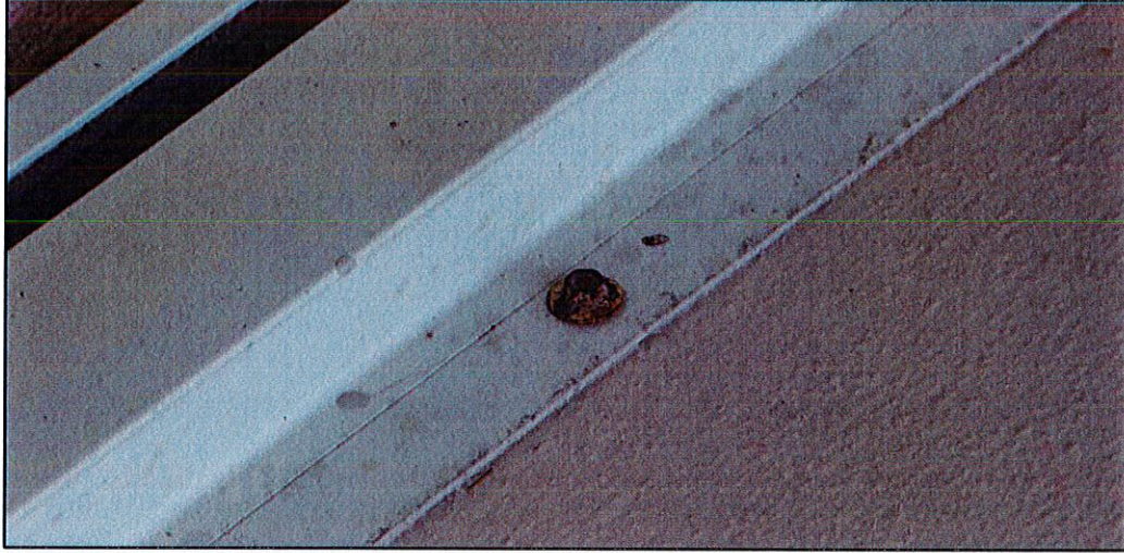
Photo #13. Close up view of deteriorated metal anchors for the hurricane shutters. (Unit 505 shown).
