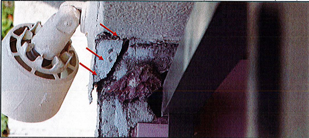
Photo #7. View of spalled concrete with observed at floor slab of unit 205 balcony.
