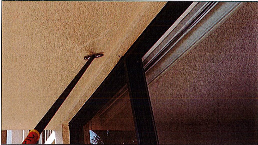
Photo #9. View of deteriorated ceiling stucco finishes, signs of concrete slab spalling due to corroded reinforcing, condition observed at ceiling of unit 204 balcony.
