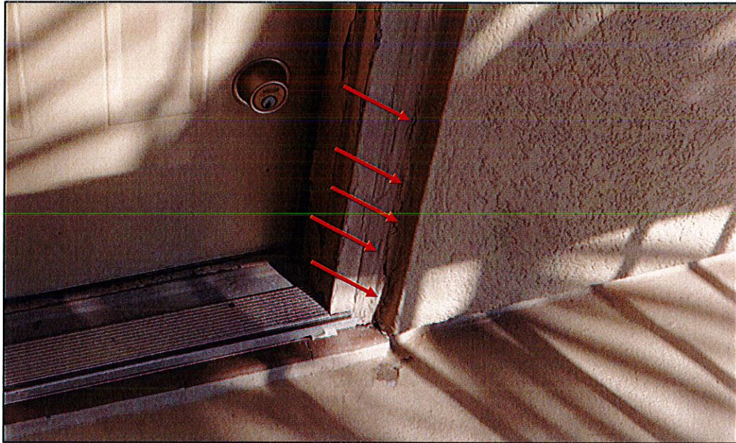
Photo #9. View of deteriorated sealant at entry door of unit 301.
