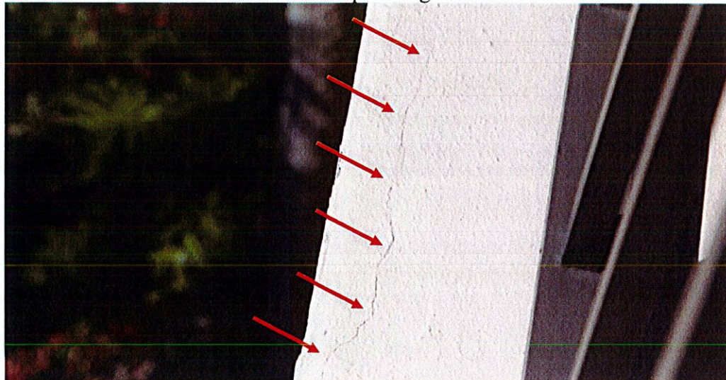
Photo #9. View of exterior unsealed cracks at edge of slab (unit 501 front corridor).
