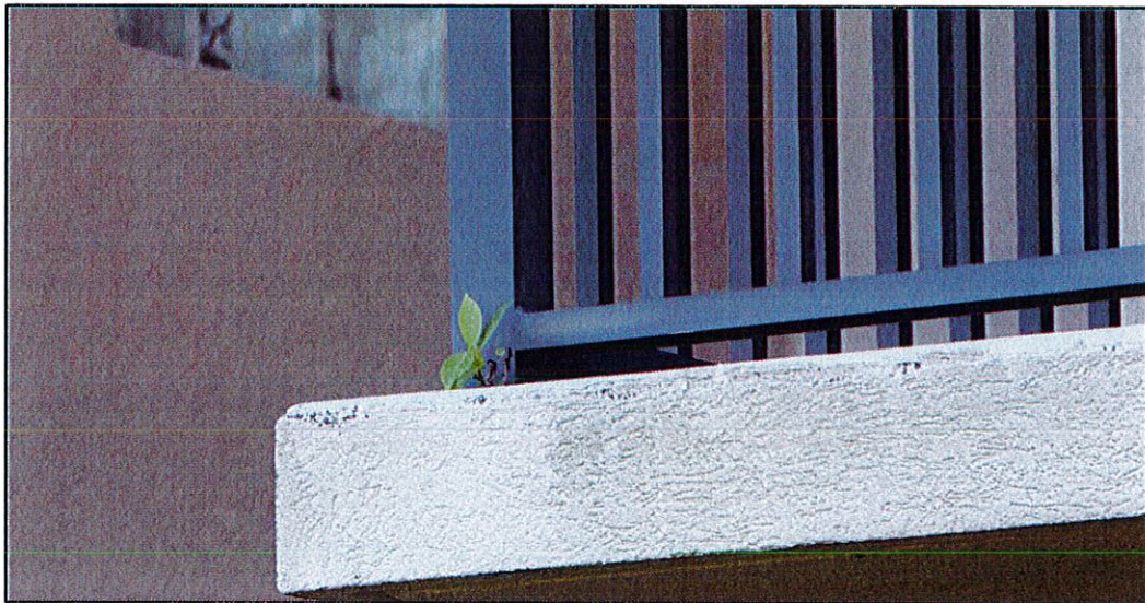
Photo #2. View of post base deteriorated grout with gaps around post and organic growth (unit 202 balcony).
