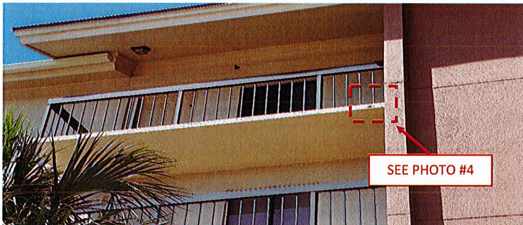
Photo #3. View of spalled concrete slab edge observed in front of unit 501.
